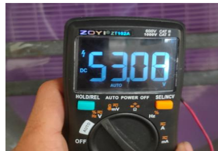
Figure 9. Generator Voltage Output Measured
