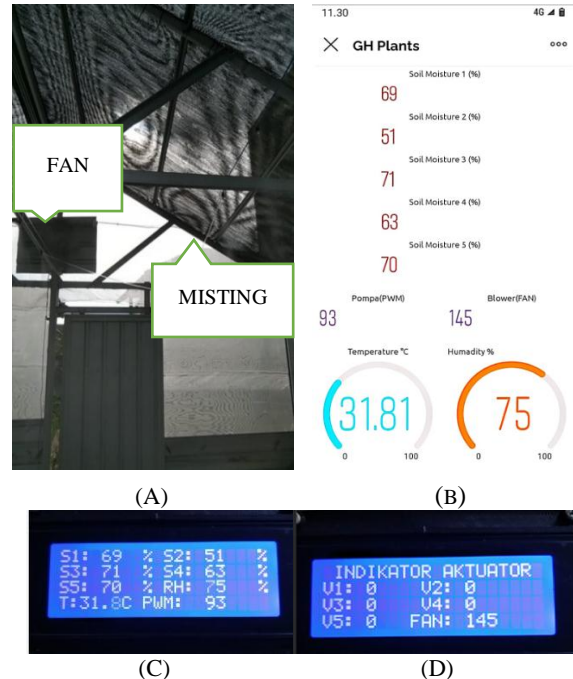
Figure 16. (A).Installation of output devices in the greenhouse, (B).Monitoring results through the bynk application, (C) and (D) Monitoring results through the actuator incubator
