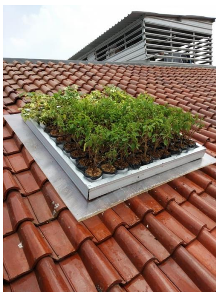
Gambar 6. Instalasi Taman Atap
